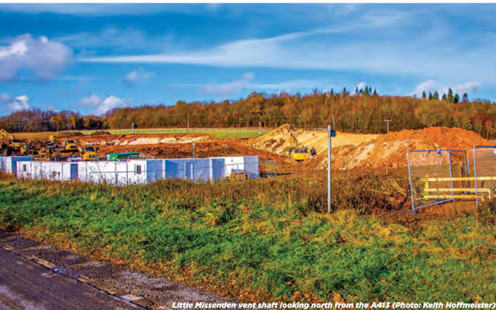
Little Missenden vent shaft looking north from the A413 (Photo: Keith Hoffmeister)
